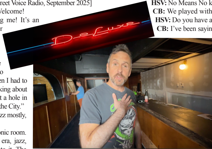
Co-owners Jay Bordeleau (L) and Christian Beaulieu (R) in the bare bones of The Deluxe. September 2025.
